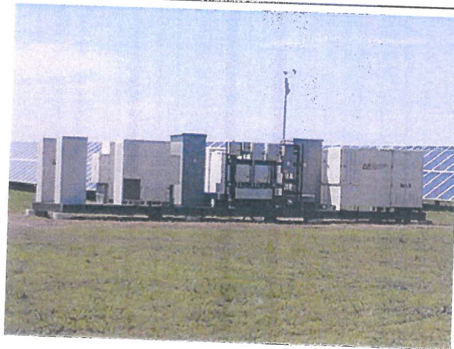
Detail of Switchgear Pad Inverters, Combiner (Junction) boxes, Disconnects Weather Station, Metering
